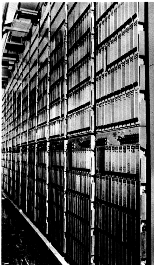
Fig. 27—REG bays, South Knoxville, Tennessee, central office.
